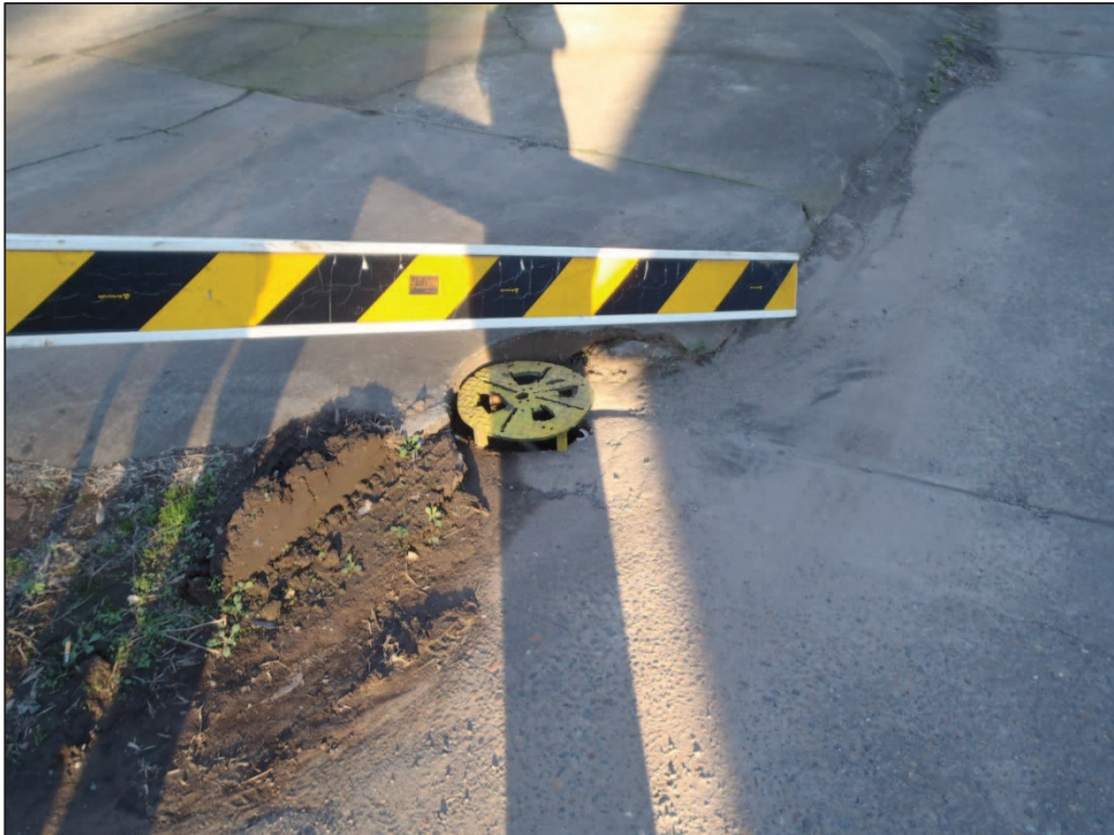
Plate 31 – Broken drain east of the Coils Factory.
