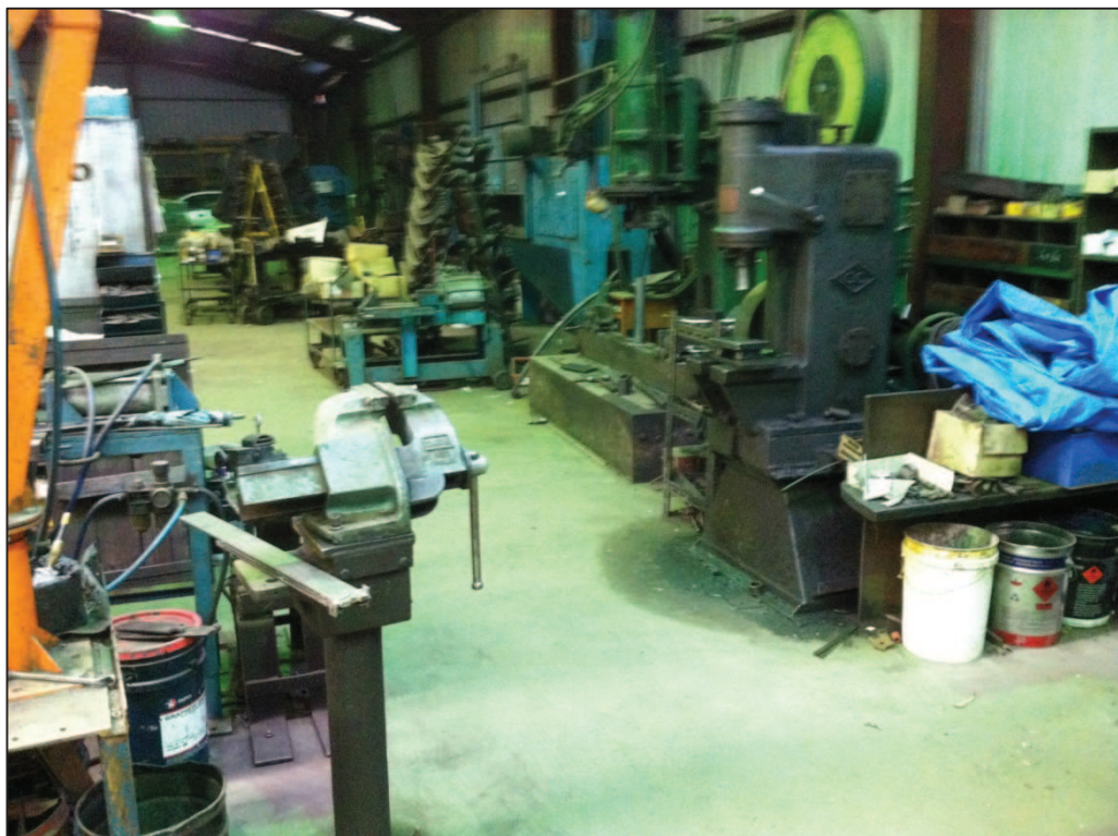
Plate 10 – Dark staining around machinery inside the Leaf Springs Shed.
