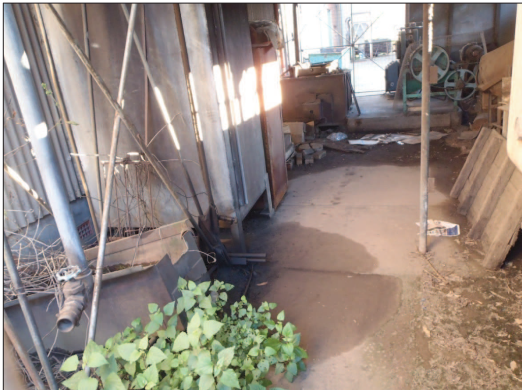
Plate 23 – Dark staining underneath AST 3 in Location 27.
