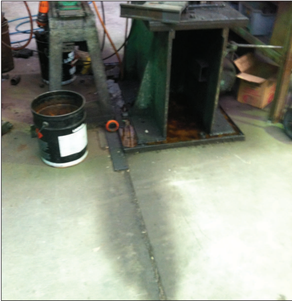
Plate 8 – Dark staining around machinery inside the Leaf Springs Shed.
